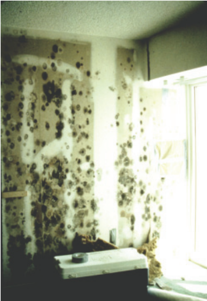
Photograph 6: Demising Wall Mold
