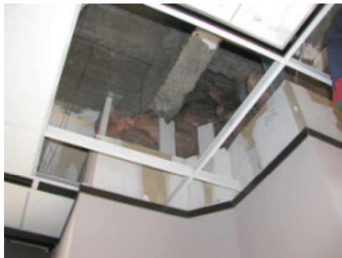
Photograph 2: Lack of Closure
